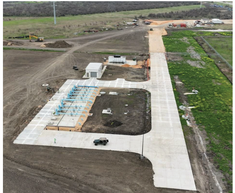
BPS – Pump Station, Electrical Building & Generator Area
