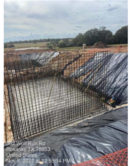
WTP/RWI - Flow Equalization Basin
